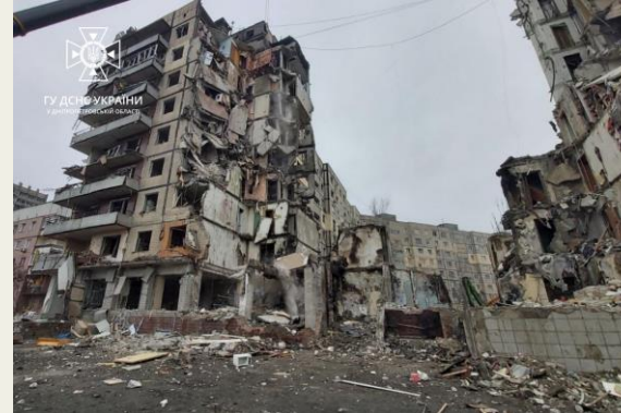
Residential complex in Dnipro destroyed by a Russian military missile attack (January 2023) [Dnipropetrovsk Main Directorate, State Emergency Service of Ukraine]
