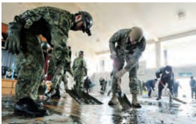
U.S. soldiers working together with GSDF troops to remove sludge from a school before the start of the new semester (Ishinomaki, Miyagi Prefecture; April 2011)
