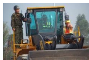
UNTPP, heavy engineering equipment training
