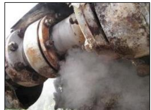
Deficiency in steam line
