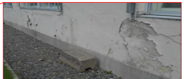
Cracks in the wall
