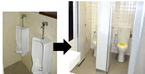
Before the renovation(male lavatory) After the renovation( Female lavatory) Improvement of section for female personnel (turning men's lavatory into women's)
