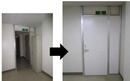
Image after the renovation Improvement of section for female personnel (barracks; installation of a door to separate section for female personnel)
