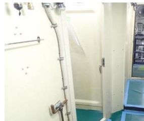
Before the installation After the installation Improvement of section for female personnel (submarines; installation of a passage door in front of the shower room)
