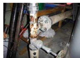
Rusty inner pipes
