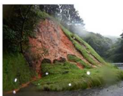
A collapsed slope
